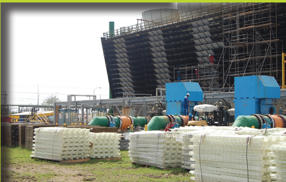
Large quantities of materials sited for the cooling tower repairs. This project is carded to be completed in June, 2012.
