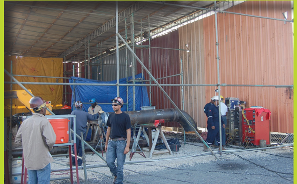
On site fabrication shop, created by DATSU, where all the piping spool pieces will be fabricated, welded, x-rayed and stress relieved before being installed for the new ammonia converter.
