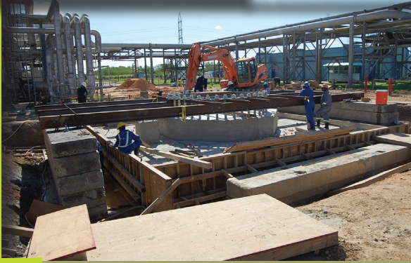
Civil work in progress for the foundation where the new ammonia converter, built in Italy, will be sited.
